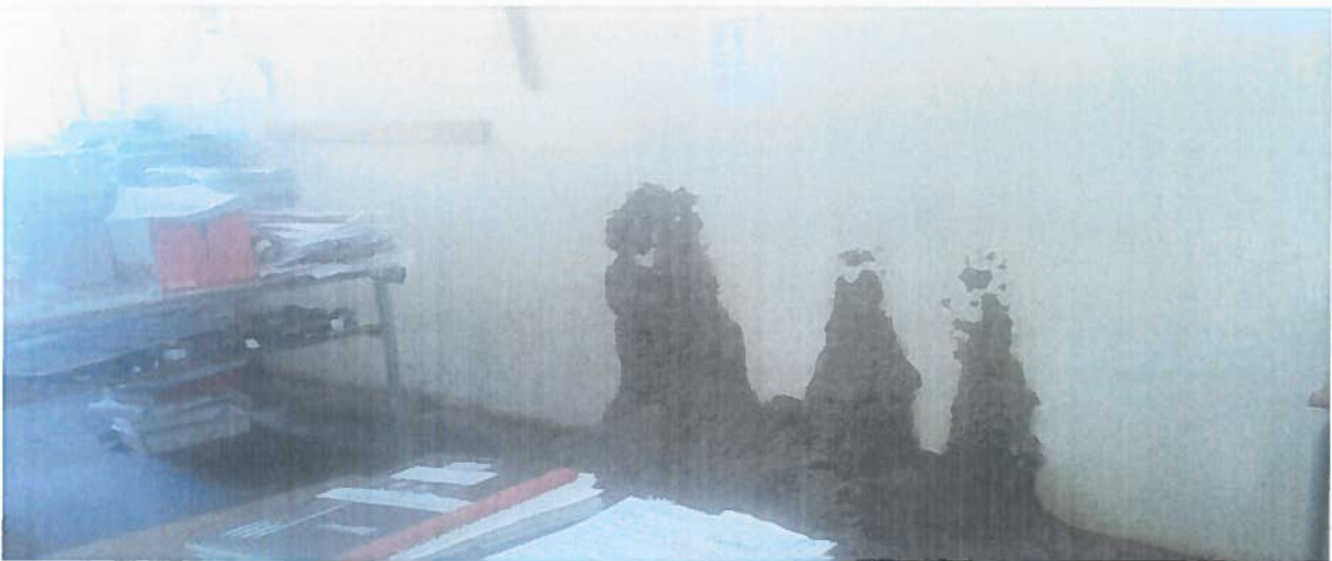
Large termite mounds in the classrooms
