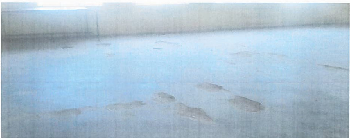
Large pot-holes in the classroom floors
