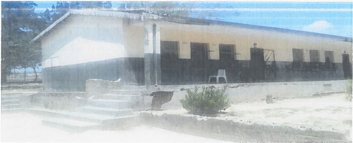
The shifting foundation of the classroom block, with gaping holes and cracks can be seen
