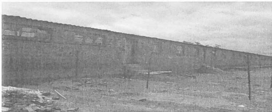
Figure 1: Old and dilapidated Hostel 1 at Sakhelwe Hostel at Kwaguqa
